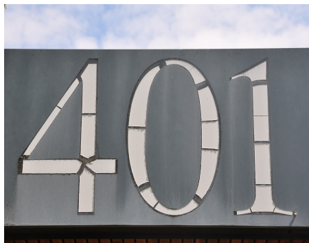
FIG. 2. Cracked lettering at Ecole Polytechnique, Palaiseau, France
